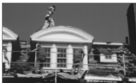
Workers under way in the summer heat, replacing shingles, and repairing dormers to the House.
