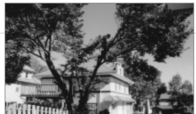
A large tree is removed from behind the house, clearing room for a new storage garage.
